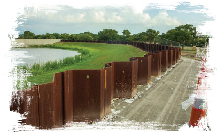
Construction to improve the Lake Pontchartrain levees. More than 350 miles of levees and floodwalls around southeast Louisiana have been built or improved since Katrina.
